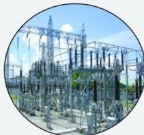
EAF Sub Station
